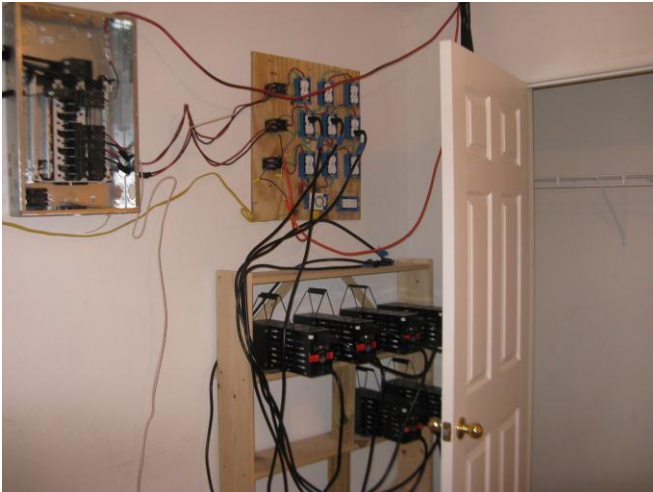
Electrical modifications to the grow room.
